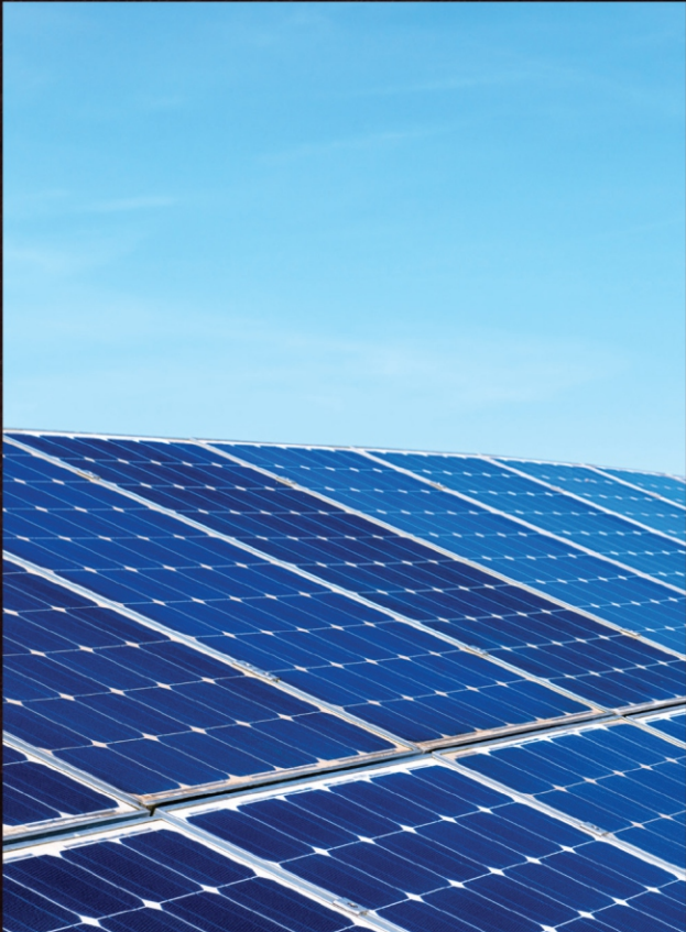
Solar Panels for Energy
